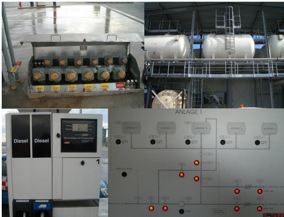
existing tank filling hose connection pit (t l), deicing tank farm (t r), fuel pump (d l), deicing control panel (d r) at Vienna Airport
